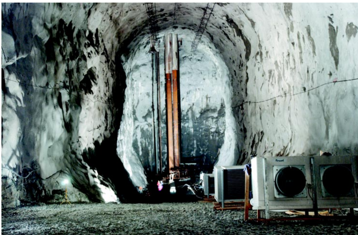
Figure 2. One of the caverns excavated in the rocks. From here, the liquid propane is pumped to the carrier vessels using submersible pumps with special motors
